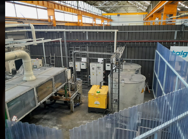
Part of Talnode®-R Pilot Plant
