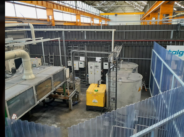
Part of Talnode®-R Pilot Plant
