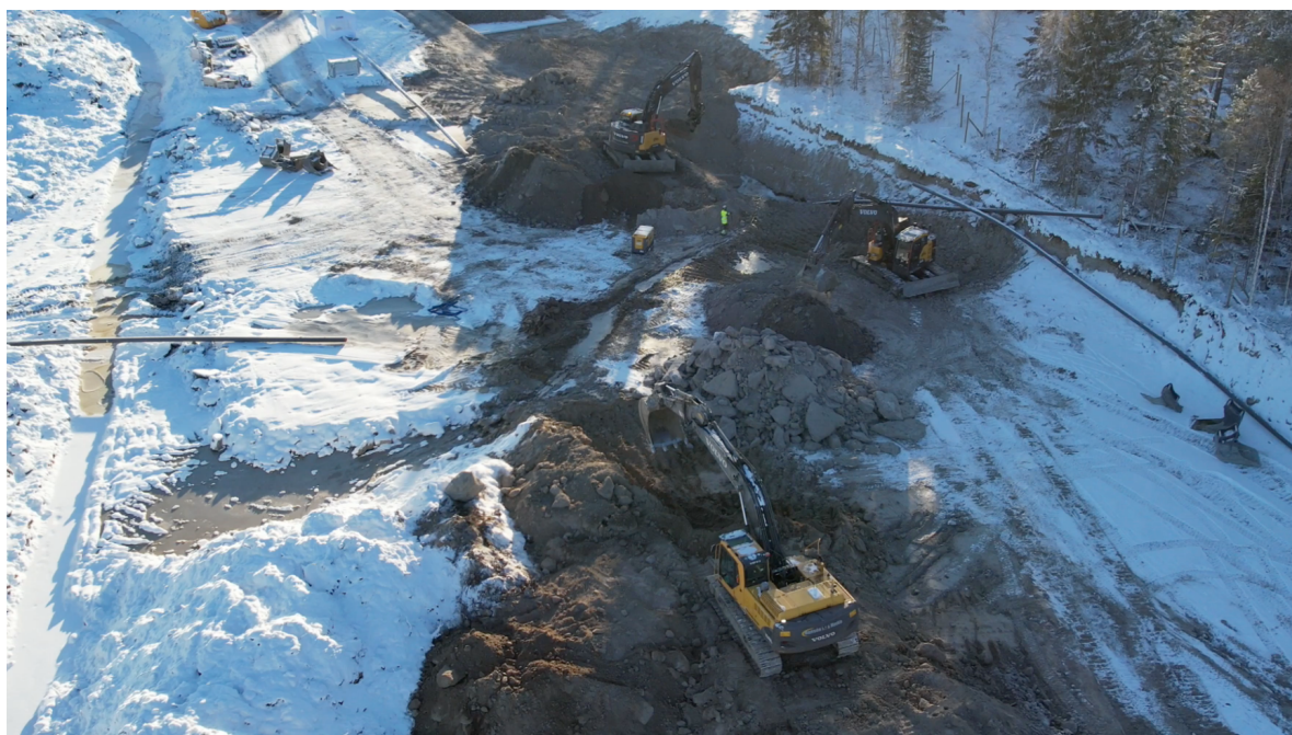
Figure 1 Stage one preparation of Talga's commercial site at the Luleå Industrial Park in Dec 2023.
