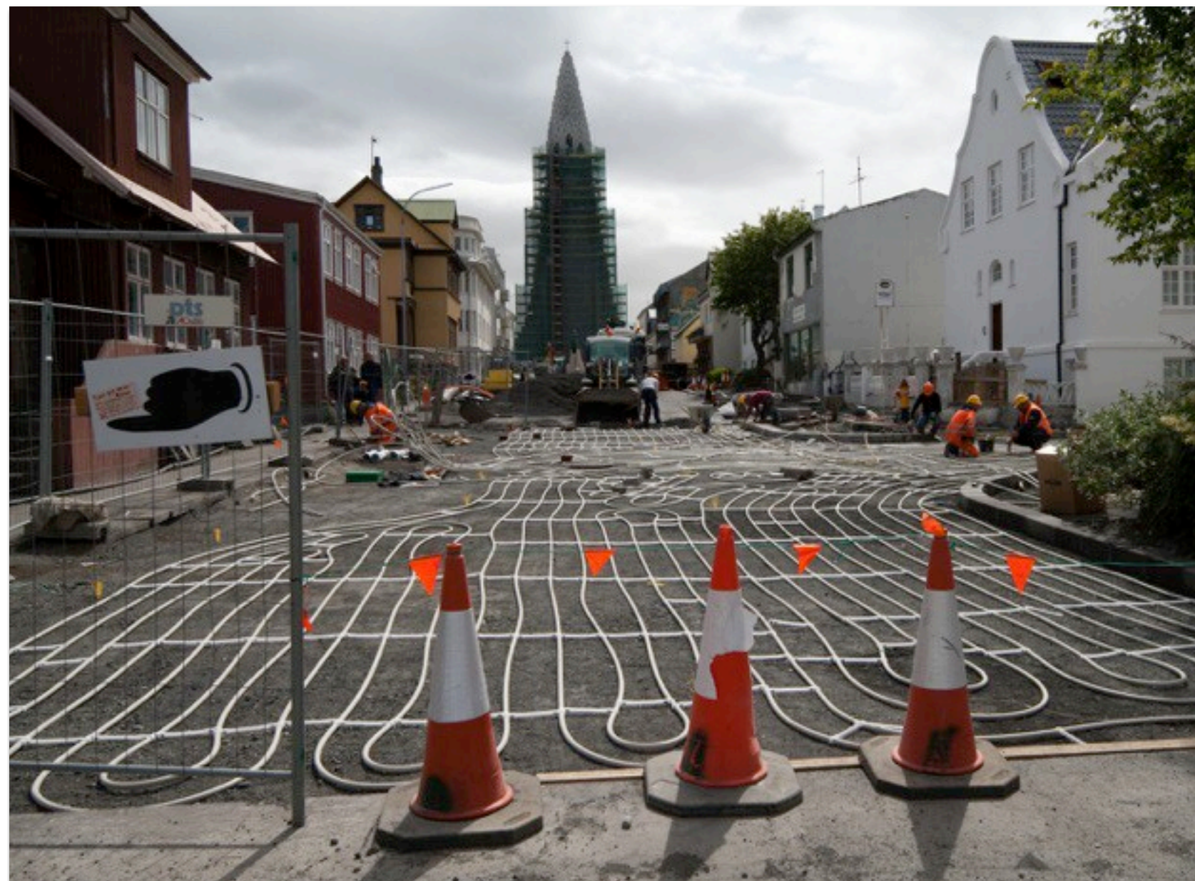
Snow & ice-free road heating installation
