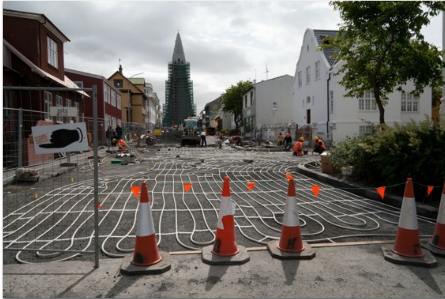
Municipal level road heating installation
