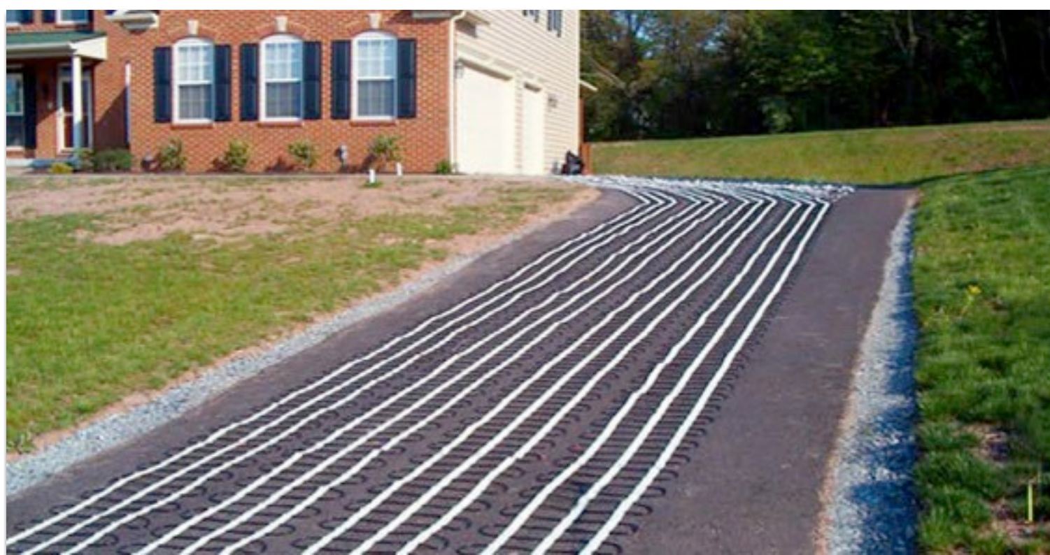
Domestic driveway heating installation
