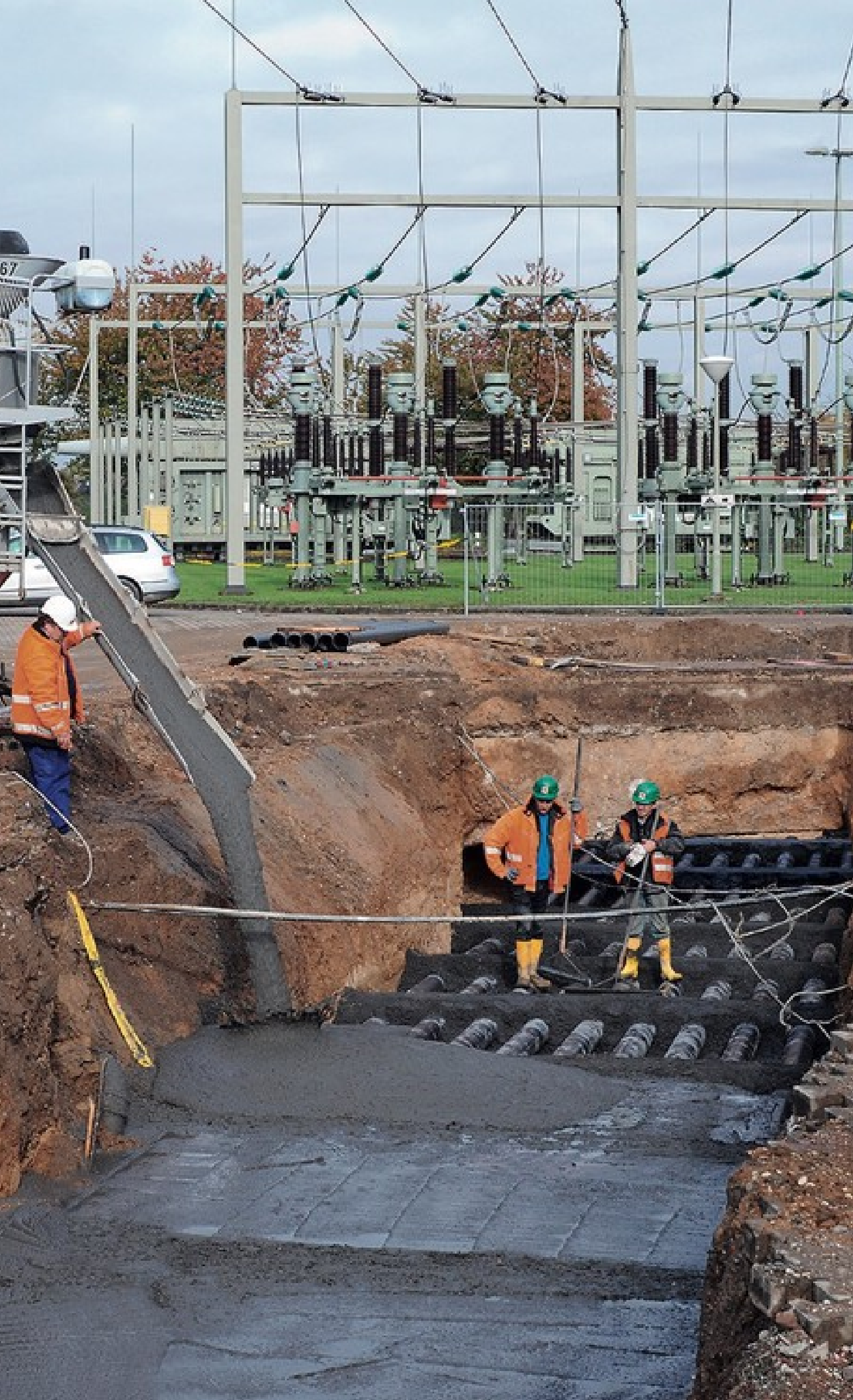
Thermal concrete in underground power line application
