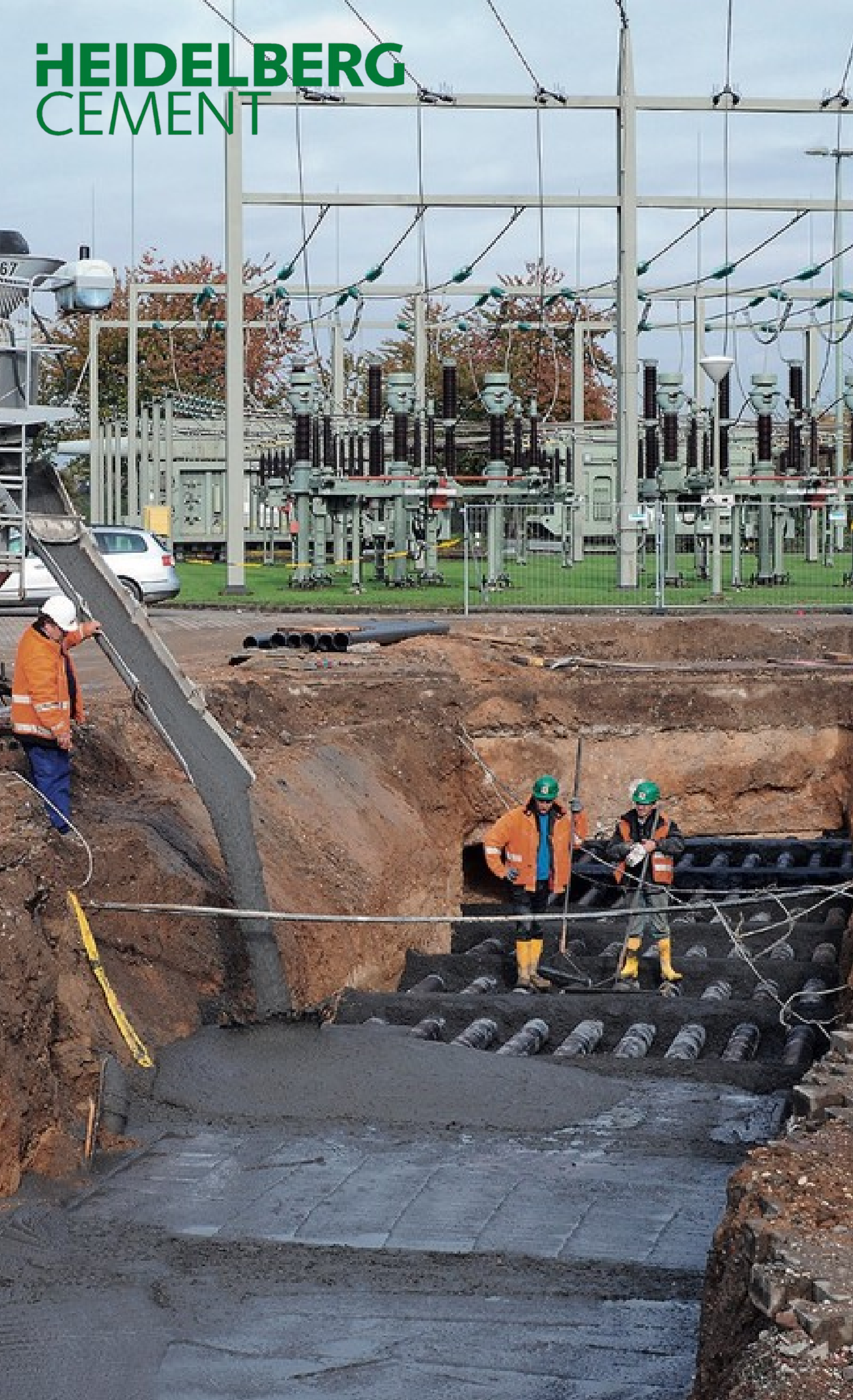
Thermal concrete in underground power line application
