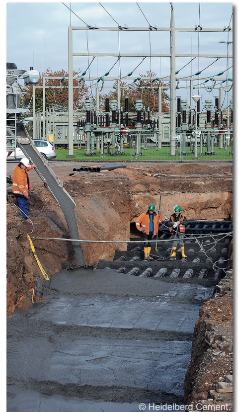
Figure 3 Thermal conductive concrete in power cable application.
