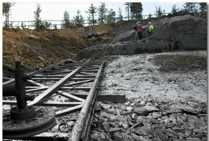
Figure 4 - Early stage of graphite ore bench development using horizontally cutting diamond wire.
